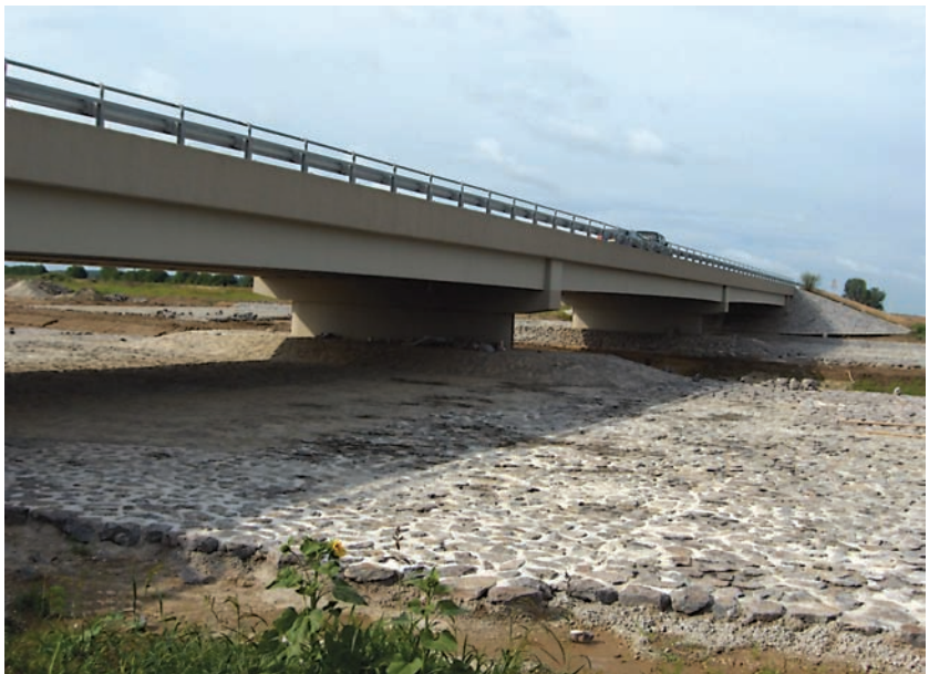
The bridge of the road No. 3804 over the inlet channel that has been raised in the course of the project
